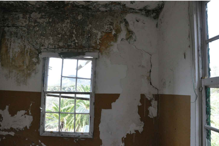
Vista interior del estado de las paredes Interior view of the state of the walls
