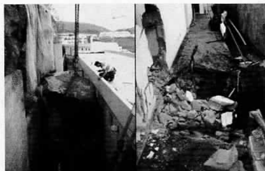
Figure 3. Removal of the 11.6 tons rock block that fell down at the back of the building. Damages caused by this rock fall.
