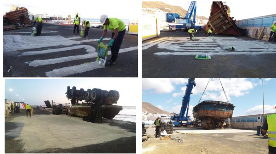
Figure 8. Sequence for the preparation of a bed of oleophilic and highly water-repellent absorbent granulates to protect the port soil and prevent water contamination.
