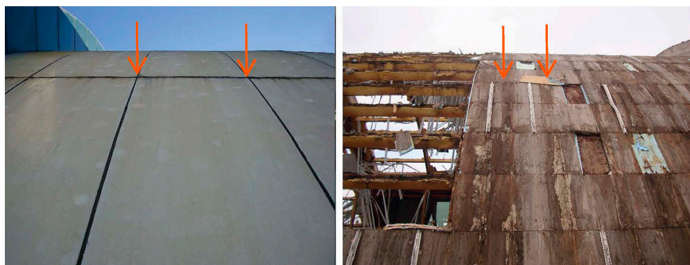
Figure 16. Left of the image: composite roof panels before demolition. Right of the image: the wooden sandwich panel during the demolition process. Red arrows indicate areas of water seepage through the composite roof panels.
