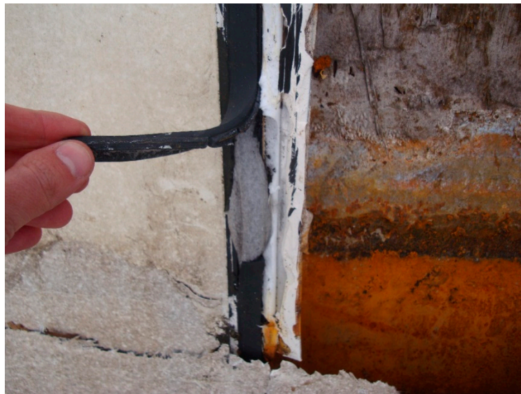
Figure 15. Aluminum omega profiles placed in the vertical joint between the composite panels. The section is filled with a foamed polypropylene as the bottom of the joint and sealed with silicone.
