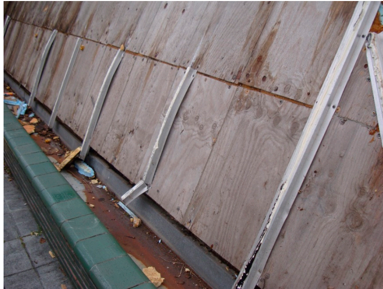
Figure 14. Aluminum omega profiles screwed to the wooden sandwich panel. Image taken during the demolition process.
