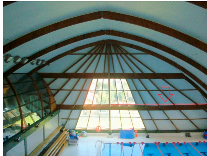
Figure 11. Deflection of a horizontal beam in the inclined façade.
