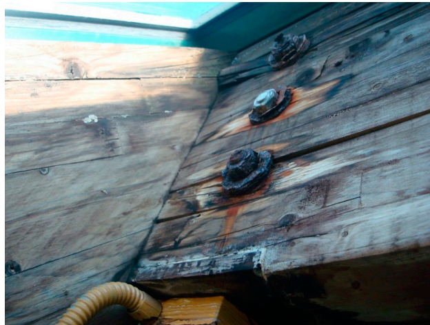
Figure 10. Corrosion of nuts, washers, and threaded rods in beam connections.
