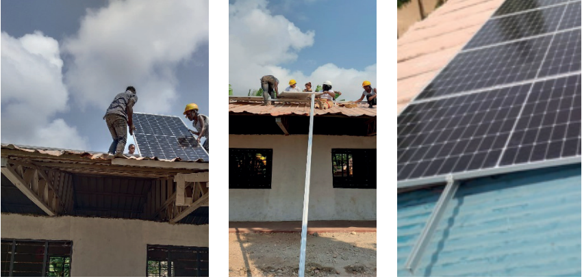
Figure 2. Installation of the solar panels on the roof of the building in progress.
