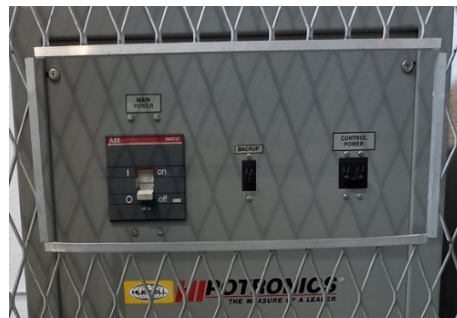
Figure 10. Power supply for the regulation of the output voltage, from 0 to 230 V.
