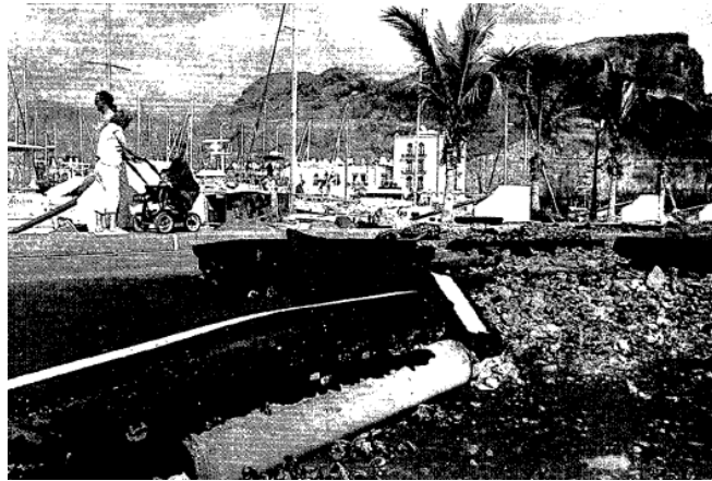
Image 3. Damage on the Puerto de Mogán road (images from "La Provincia").
