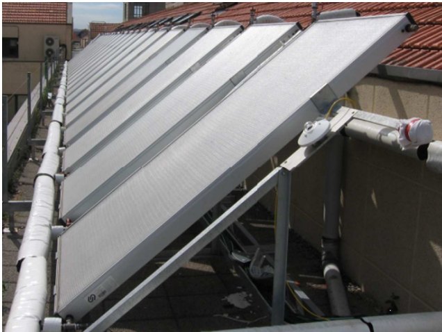
Fig. 1 Photograph of the solar thermal collectors located in the upper part of the East Department Building at the University of Oviedo.
