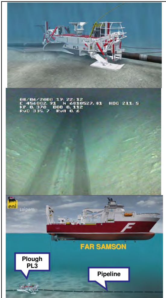
Fig.10 Part of the animation showing the process of how the PL3 places pipelines onto the sea bottom.
