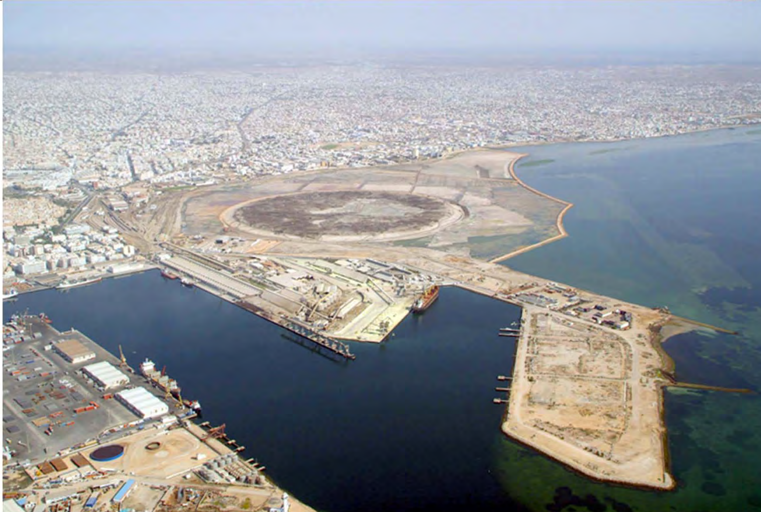
Remediation and rehabilitation works at the north coastline of Sfax – Taparura project (Tunisia) | 2006-2009
